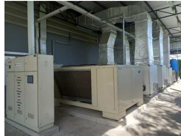
Air Control System
